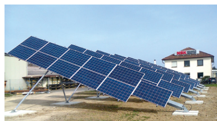
Solar panels at Neuwig
